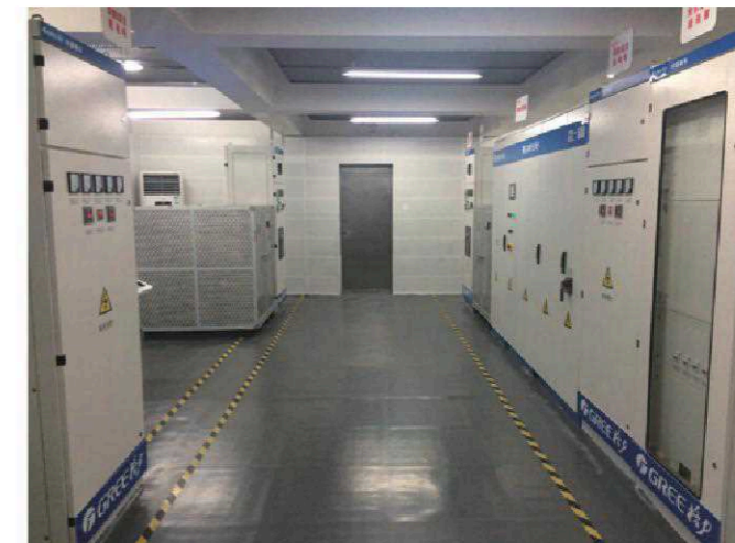
PV Power Room
